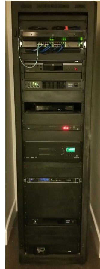
Typical Boardroom Rack
